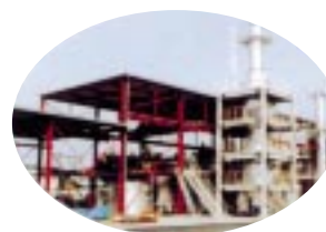
JAMA R&D experimental facility for waste gasification.
